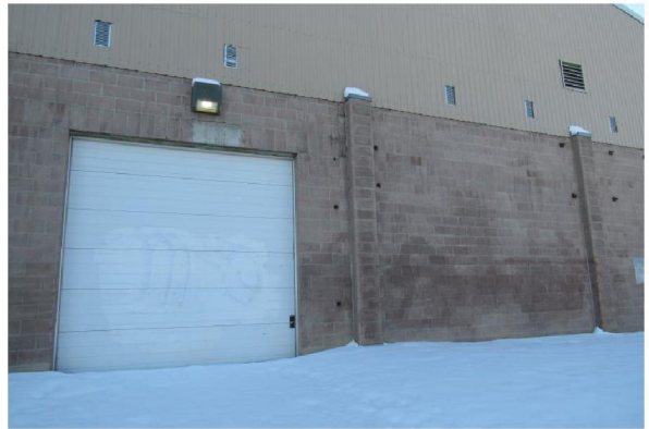
Photo #E8: Exterior LED light.
