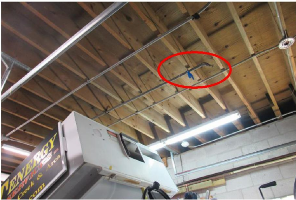
Photo #M11: Wet pipe sprinkler system in Zamboni room.
