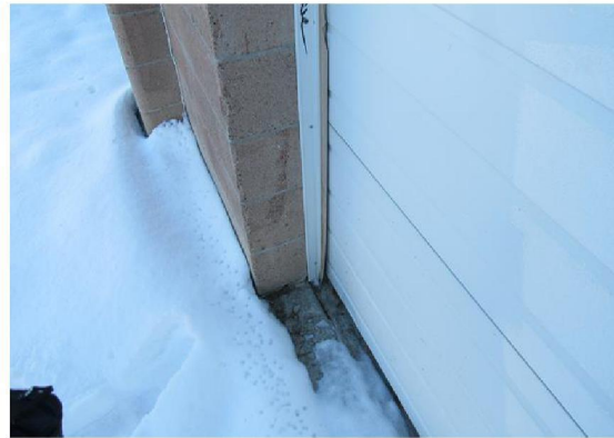
Photo #A8: Improper sealant (weather stripping) shown at the overhead door on the rear of the building.
