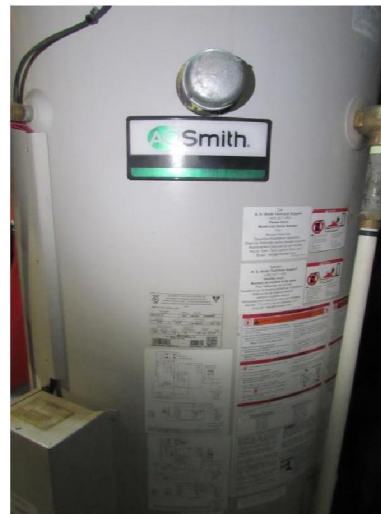
Photo #M10: AO Smith water heater.
