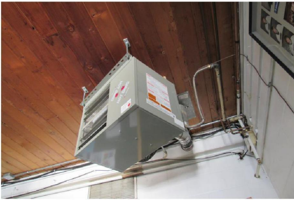
Photo #M5: Ceiling mounted radiant heater.
