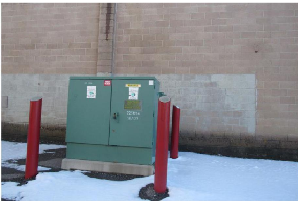
Photo #E1: On site electrical transformer.
