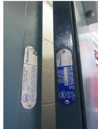
Photo #A16: Interior fire rated door.
