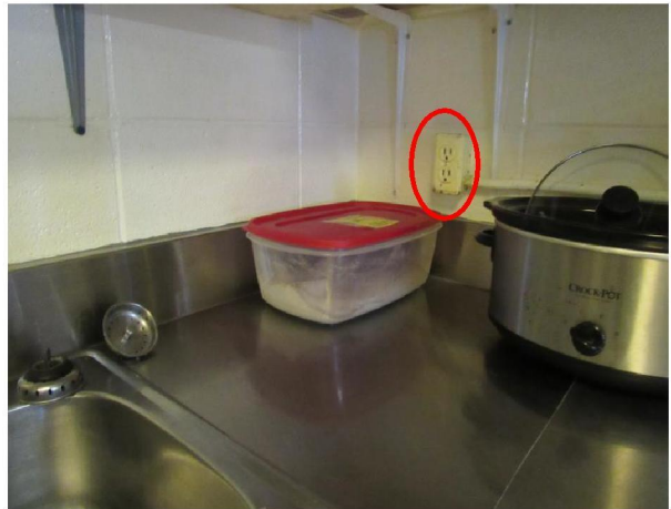
Photo #E6: Non GFCI receptacle found within 1 meter of a sink.
