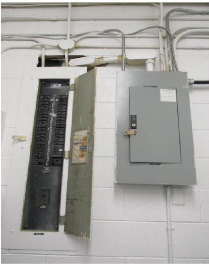
Photo #E5: Subpanels located in referee room.
