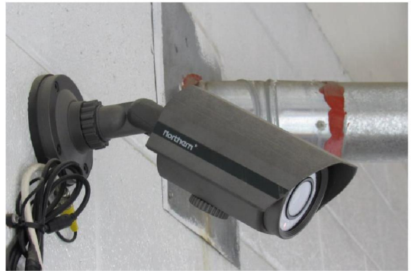
Photo #E10: Northern surveillance camera
