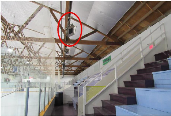
Photo #M7: Overhead electric radiant heaters.
