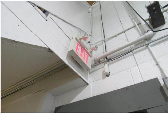
Photo #E9: Exit and emergency lighting.
