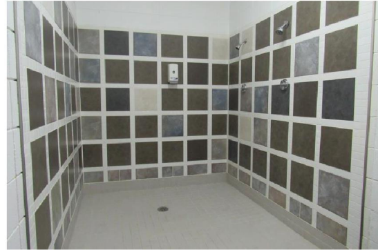
Photo #A14: Ceramic wall and floor tiles in change room shower area.
