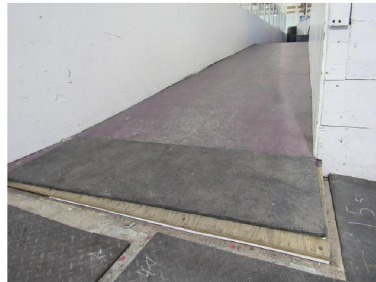
Photo #A18: Tripping hazard and lack of handrails on barrier free ramp near bleachers.
