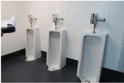
Photo #A17: Urinals located in main lobby washroom; not barrier free compliant.
