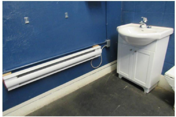
Photo #M6: Hydronic baseboard heater.
