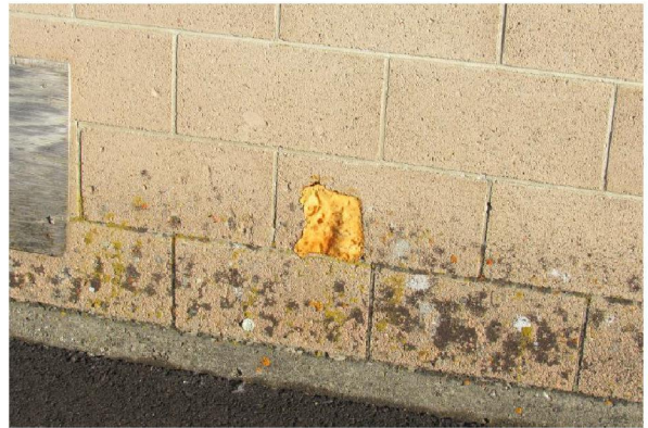
Photo #A6: Previous fix in cladding exposed to elements.
