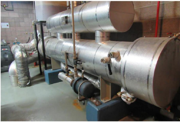
Photo #M13: Ice plant chiller/heat exchanger.
