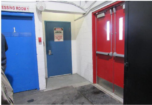
Photo #A15: Ammonia plant entry and utility egress doors.
