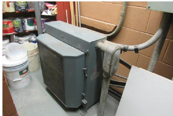
Photo #E2: Interior transformer.
