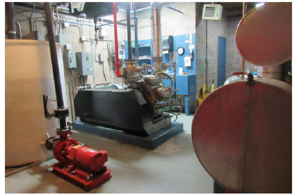
Photo #M18: Compressor and circulation pumps in ice plant.
