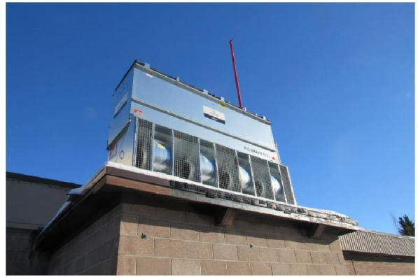
Photo #M14: Cooling tower for ice plant.
