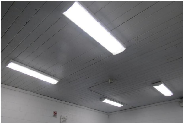
Photo #E7: Ceiling mounted fluorescent lights.
