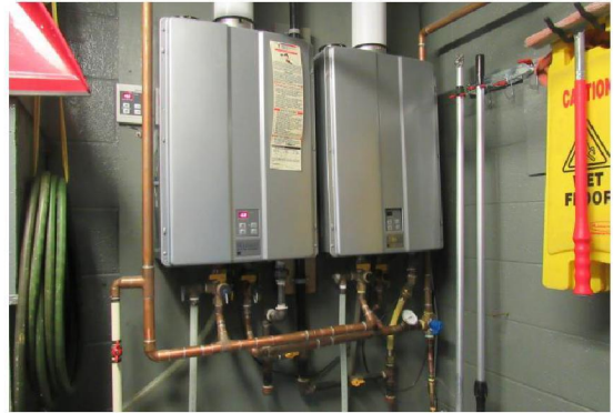
Photo #M8: RINNAI instant hot water heaters.
