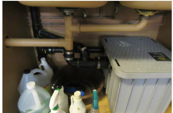
Photo #M2: Grease trap and piping.
