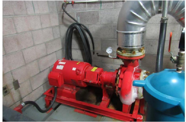
Photo #M16: Brine Pump.
