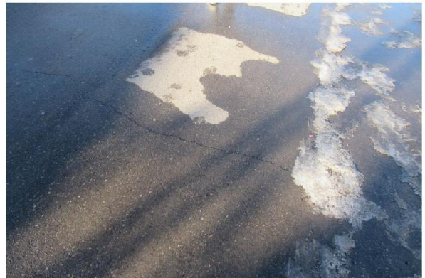
Photo #A2: Asphalt Cracks in parking lot.
