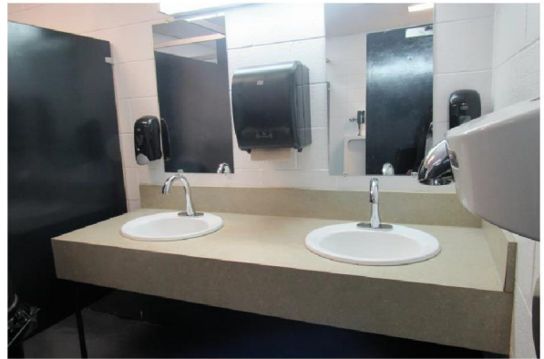
Photo #M4: Counter mounted sinks in washroom.
