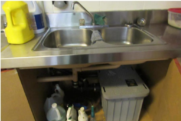
Photo #M1: Stainless steel double basin sinks in canteen.
