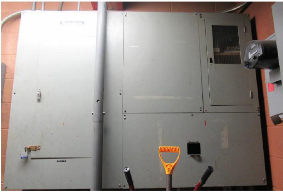
Photo #E3: Central distribution panel/switchgear.
