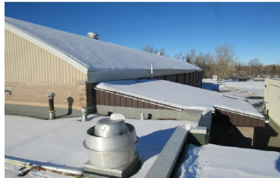
Photo #A20: Cap flashing and SBS arched roof and asphalt shingle sloped roof.
